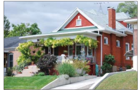
This porch has been altered and, as a result, this aspect of historic character has been compromised.
