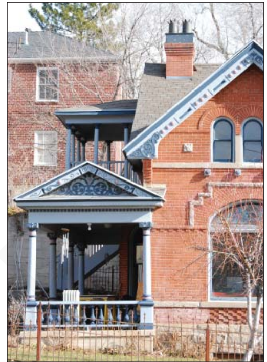
Maintaining the composition and embellishment provided by original architectural detail is essential.
