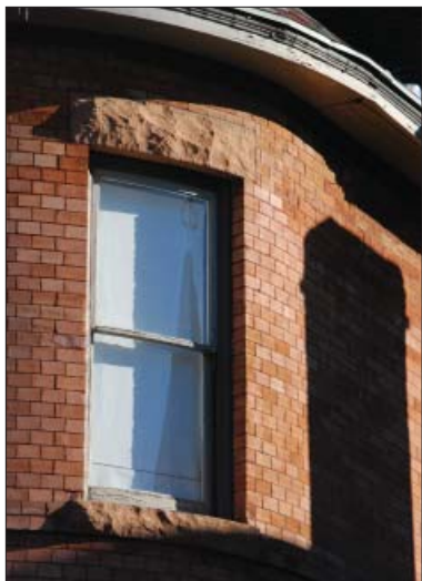
The appearance and integrity of the original masonry can be successfully maintained through appropriate repair.
