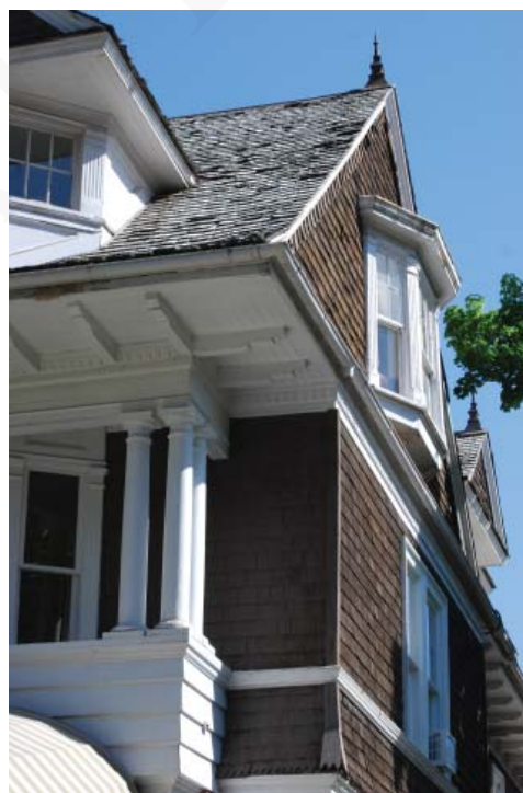
Wood shingles unify both walls and roof, concentrating visual texture as a background to Classical detail.
