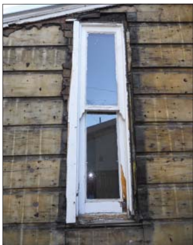
Removing later materials may reveal the original materials, such as this siding, which with care can be successfully repaired.
