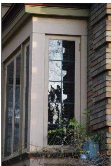
Framing sections, profiles and materials define the type of window and add considerable detail to the facade.
