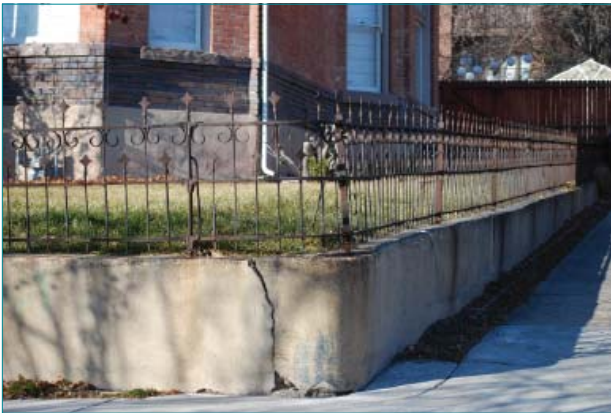
Cast and wrought iron railings with low concrete retaining walls are still a characteristic streetscape feature, defining public and private, while providing decoration and maturity.
