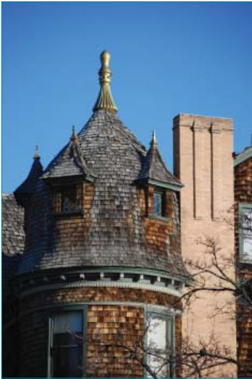
Due to the large size of many of the buildings in the district, roof materials are very important visual features.
