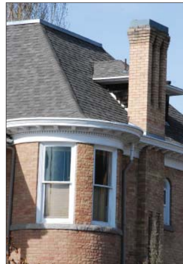
Asphalt shingles are the typical and appropriate roofing material for this style and period of architecture.
